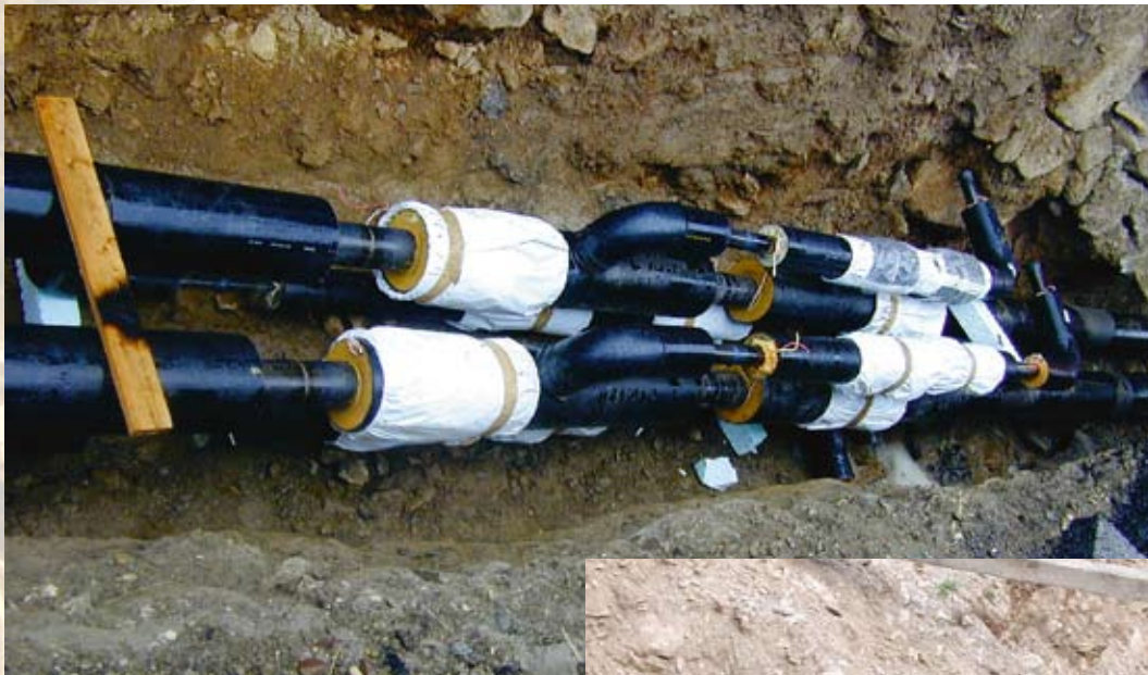
Underground pipes for a district heating system. In this case, the supply and return-flow pipes are individually insulated.
